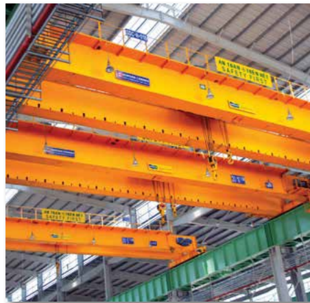
Double Overhead Hoist Crane
