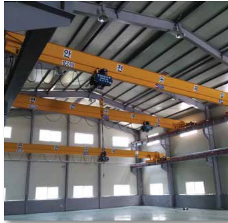
Single Overhead Hoist Crane
