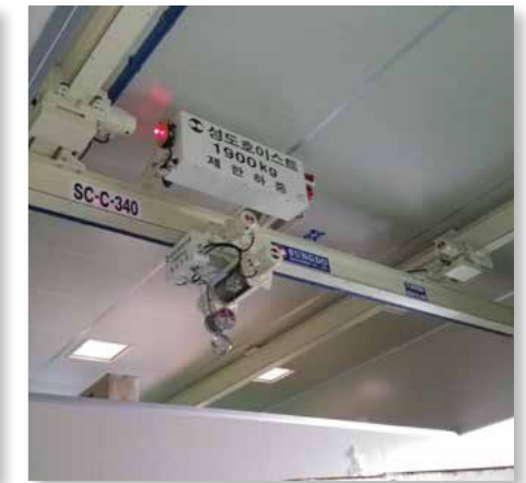
Clean Room Hoist Crane
